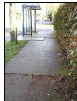
Dilapidated sidewalk eastside of Milwaukie Ave. at bus stop
